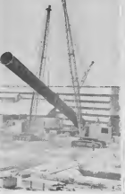
The stack, undisturbed from its base, is slowly lifted by two crawler cranes. A third crane (picture 3) lifts the bottom.
